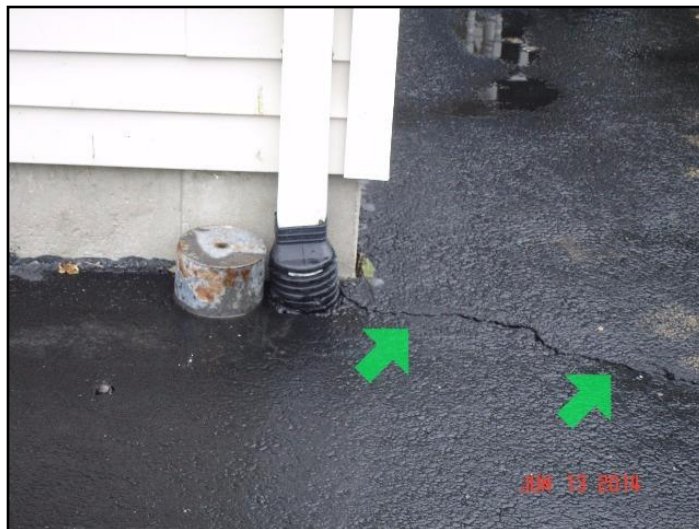
23. Cracked or damaged surfaces
