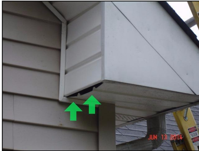
21. Loose or missing pieces
