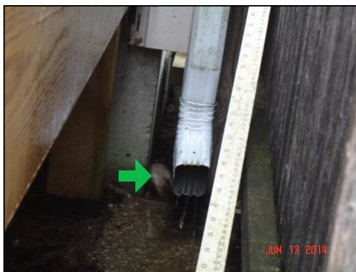
1. Downspouts end too close to building
