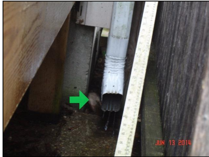
20. Downspouts end too close to building
