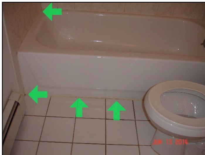
10. Caulking loose, missing or deteriorated
