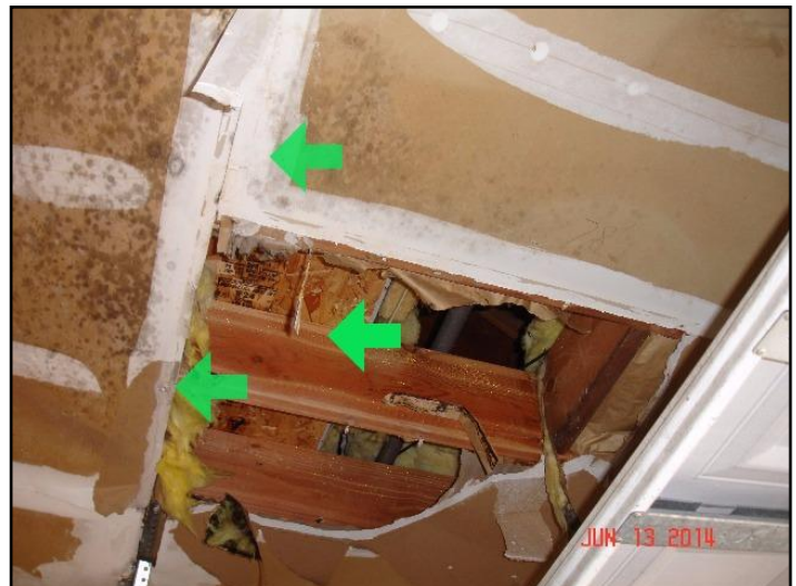
53. Stains Possible leak
