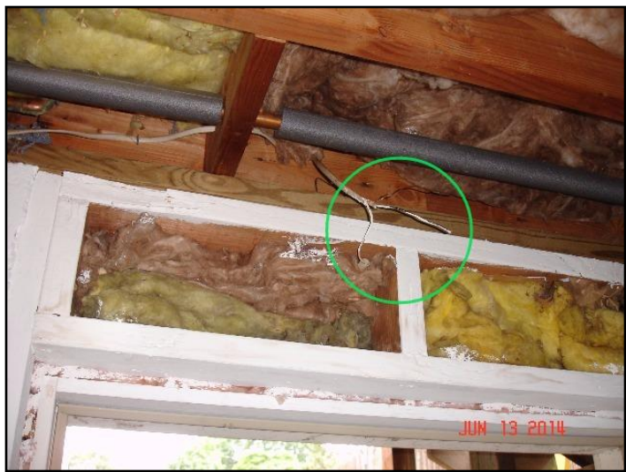
38. Exposed on walls or ceilings
