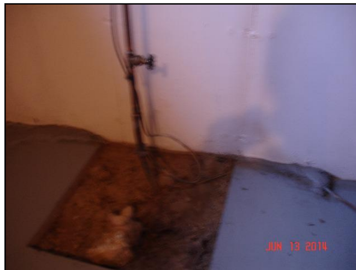
33. Copper - water pipe
