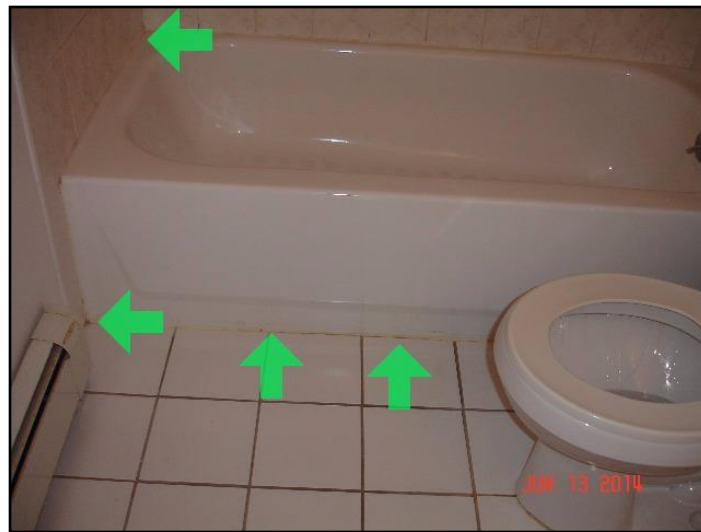
49. Caulking loose, missing or deteriorated
