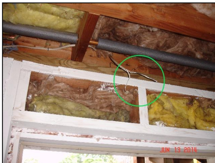
6. Exposed on walls or ceilings
