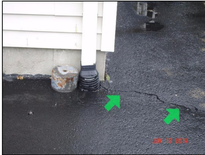
3. Cracked or damaged surfaces
